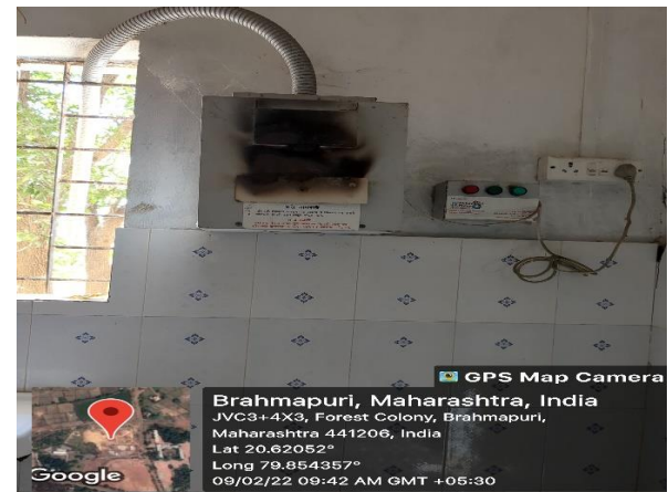
Sanitary pad Incinerator
