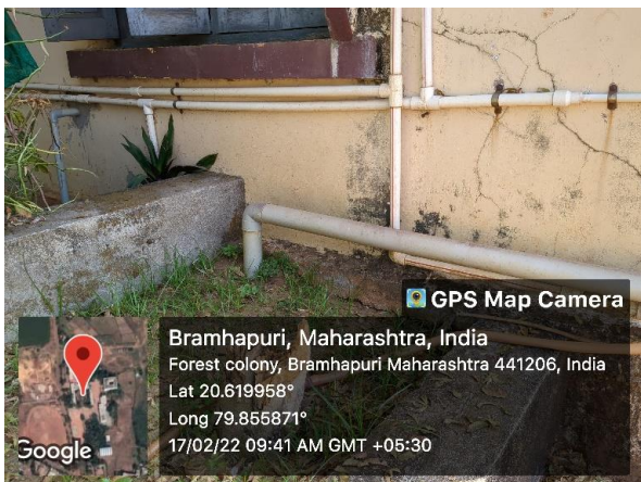
Sewage Line for Laboratory Waste
