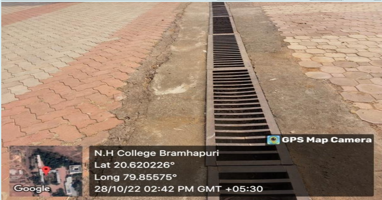
Water canal attached to the Rainwater Harvesting Sites
